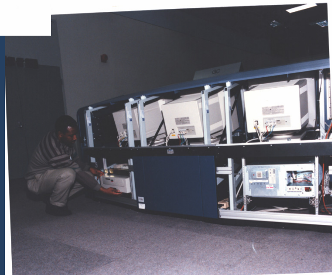
Workstation level maintenance in new control center
